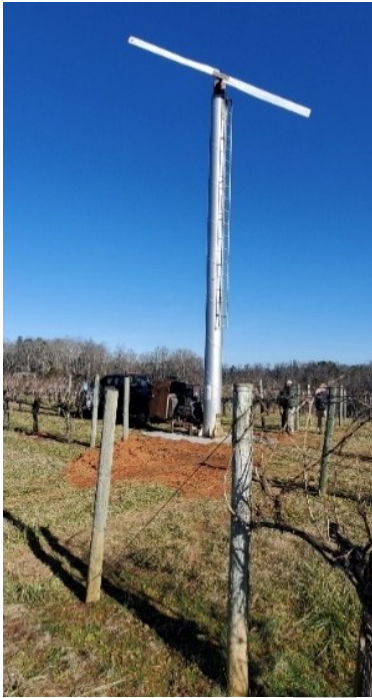
Figure 2: A stationary wind machine in North Carolina. (Photo: Eric Case)
